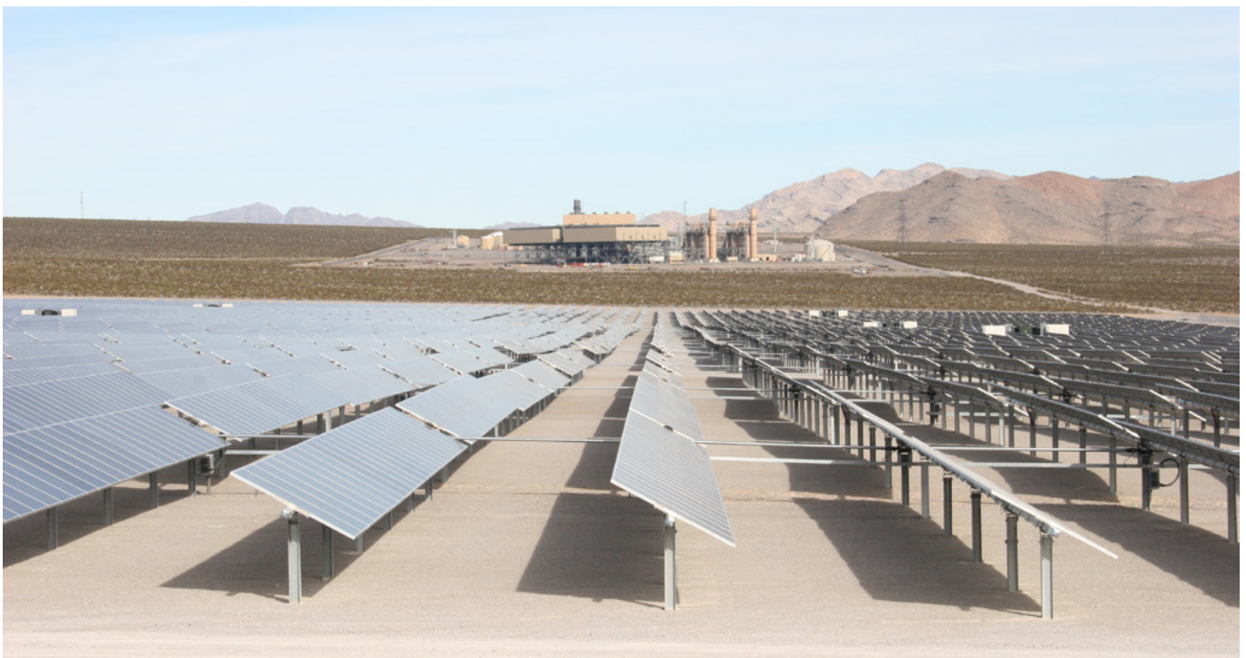
Figure 1. A 20 MW capacity "Sun Machine" solar farm is shown in foreground, associated with the background 585 MW gas turbine combined cycle power plant at the Silverhawk Generating Station, in Las Vegas, Nevada 5 .
