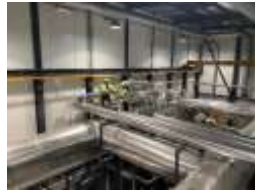
Counter Flow 2 stage 1,200 kW HRSG 11 Bar steam with water pre-heater on Hydrogen plant
