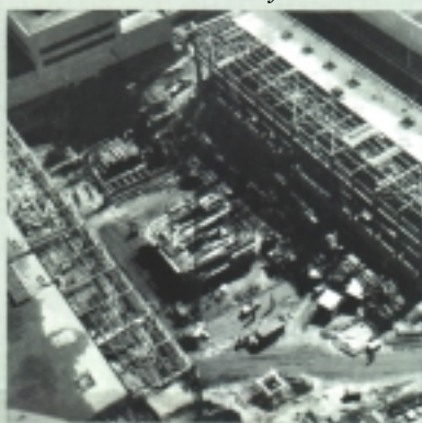
An April 1953 aerial of partially completed 50,000-ton press foundation (center) and excavation and cofferdam for 35,000-ton press nearby. Forge shop extension (left), pump station (right) under construction.
