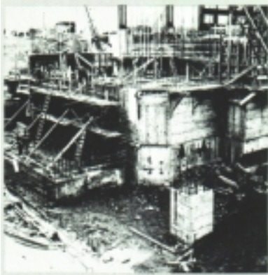
Lower part of 50,000-ton press foundation, some 100 feet below floor level to bedrock.
